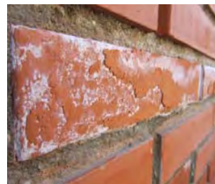
Efflorescence and Spalling
