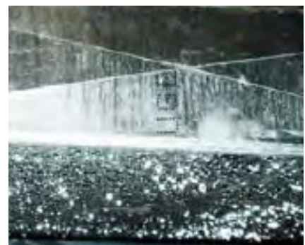
Duct condensation heater
