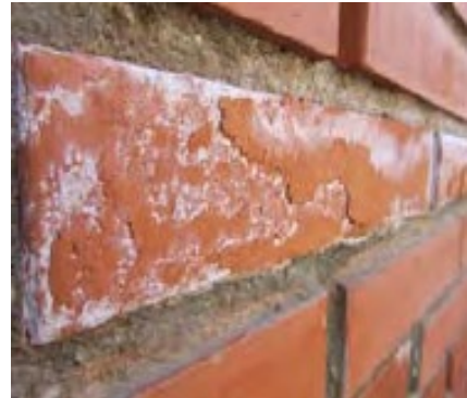
Efflorescence and spalling
